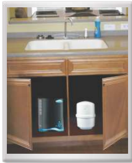
Customized placement of the filter below the counter with the tank to suit the space.
